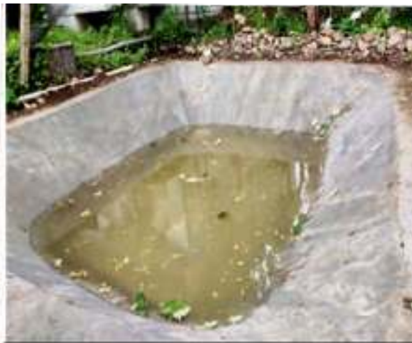
Coconut coir Cement Tank
