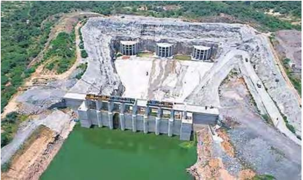
Palamuru-Rangareddy Lift Irrigation Scheme has been built on the Krishna at a cost of ₹35,000 crore in Nagarkurnool district. (HT Photo)
