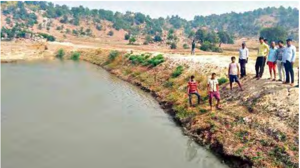
A check dam built by villagers along with Maghadh Jal Jamaat near Sijuaghati in Imamganj-Dumaria area.
