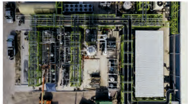
The ZwitterCo membrane skid is in the bottom middle-left of the Solugen chemical manufacturing factory
