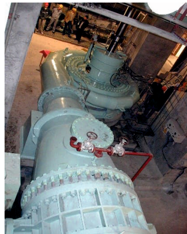
The view of Metallic volute pump of 5 Cumecs flow with 130 M Head and driven by 8500 KW electric motor.
