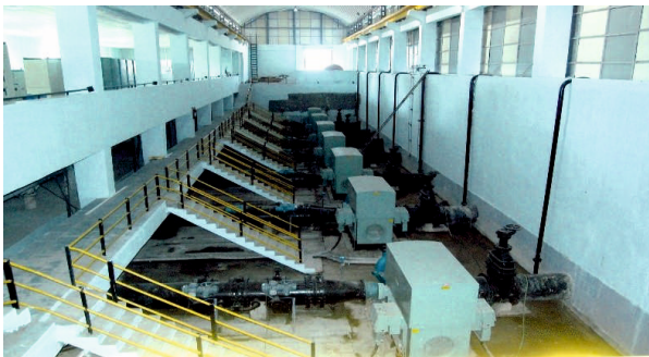
Photographs of the pumping stations
