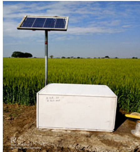
Prepaid Metering system installed in farm
