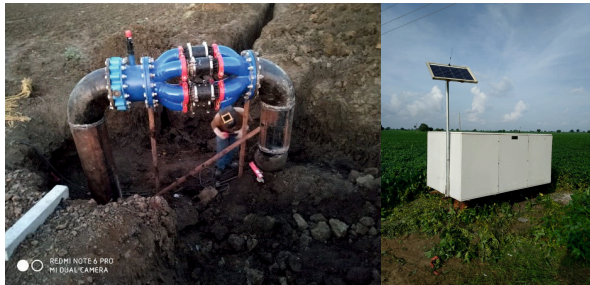
Sabotage Management System installed in the field.
