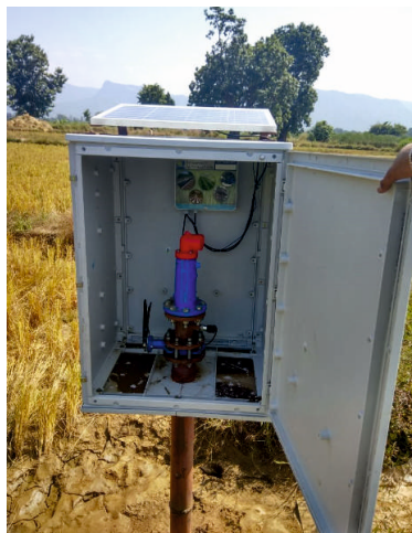
Air Management system is installed on pipe line to monitor pressure
