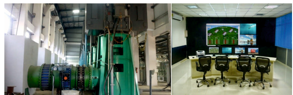
Pump house and Central Control Room
